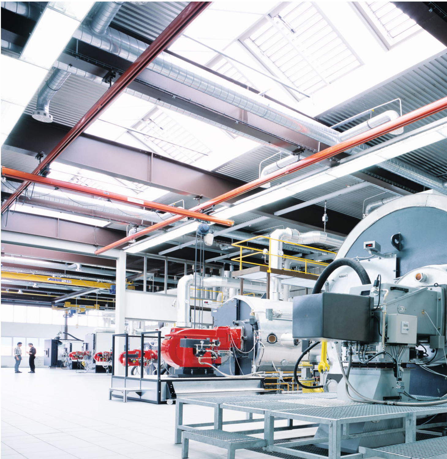
Test firing chambers at the Weishaupt Research & Development Centre
