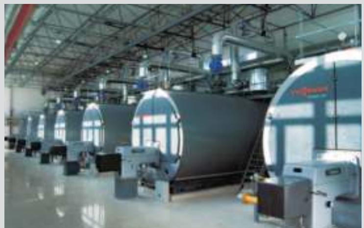
Xi'an, central China: The seven WKG gas burners in this heating centre provide more than 50000 residents in the Zi Wei garden district with 115 MW of heat
