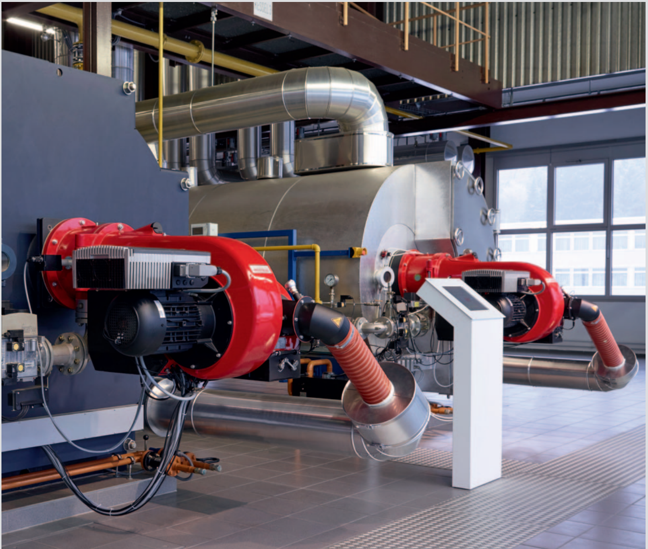
Burners with FGR on long-term test in the Weishaupt factory's boiler room
